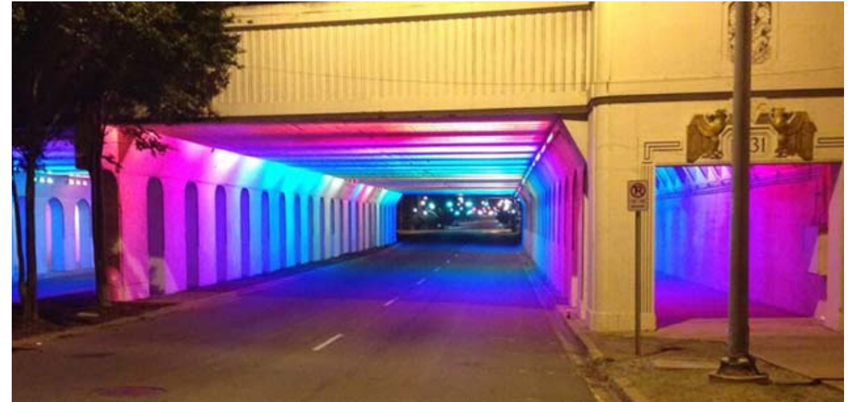
Bridge viaduct lighting can improve safety while providing an artistic element in an underutilized space.
